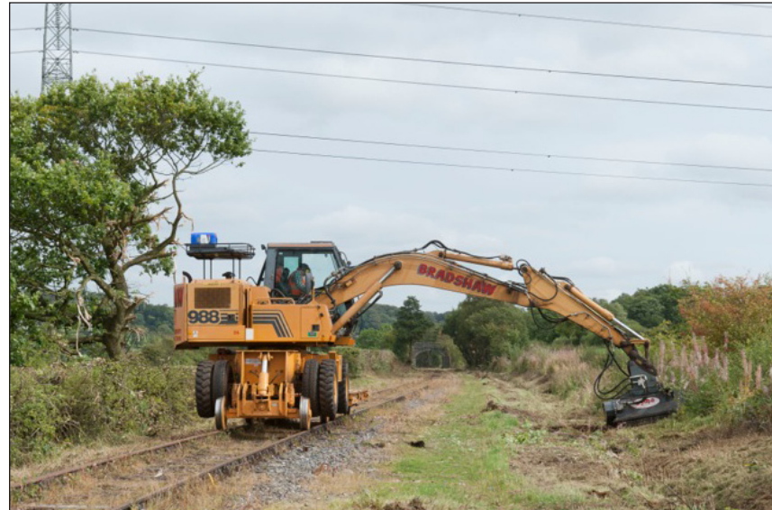
▲ Work takes place between Denford and Endon to clear the first section of the route between Leekbrook Junction to Endon. David Gibson
